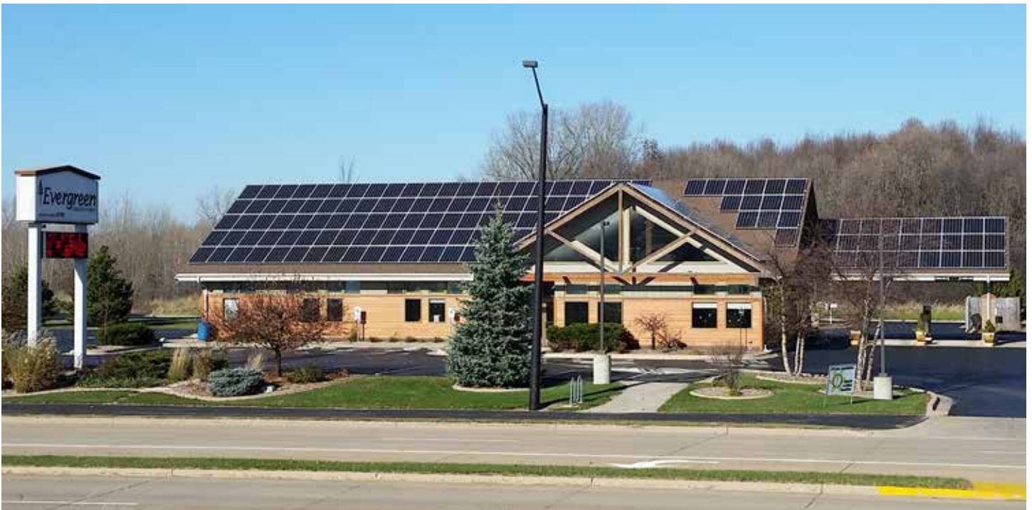
Solar array installation complete in November of 2015.
